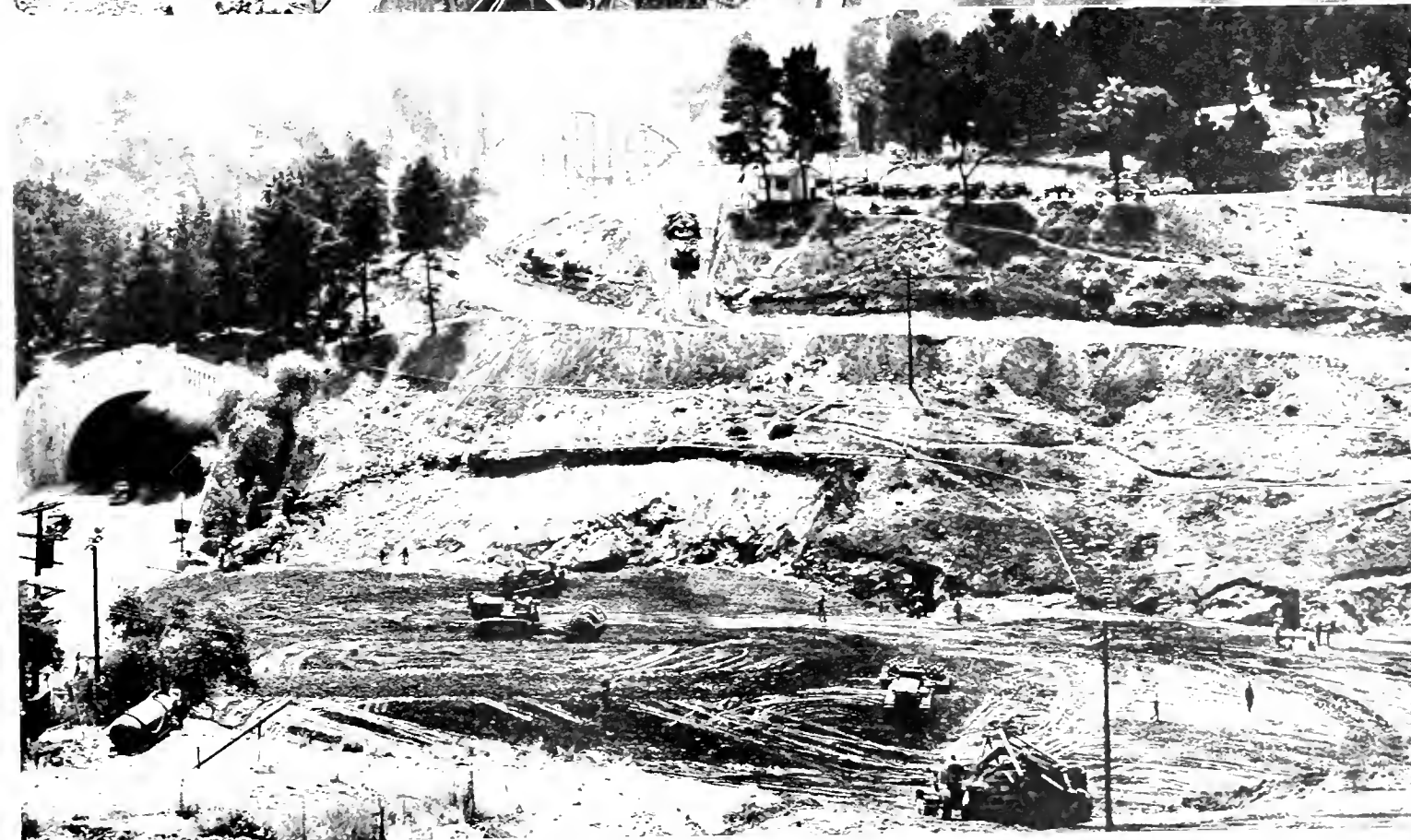
Top view shows existing Figueroa Street tunnel on right and construction at Solano Street grade separation with Park Lane bridge in background. At bottom—Extensive grading at site of Bishops Road grade separation and construction of dam that will also serve as highway embankment. Excess excavation material is used for dam which permits extension of city-owned reservoir
